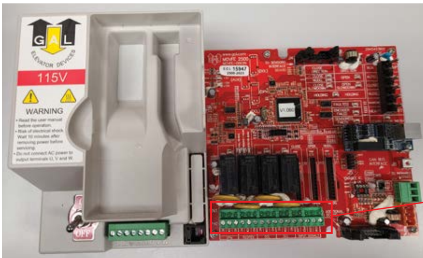
Existing 16-pin connector. To be replaced with wiring harness.
